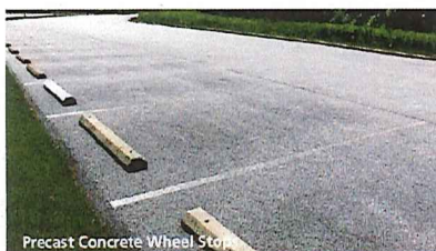
Precast Concrete Wheel Stop
