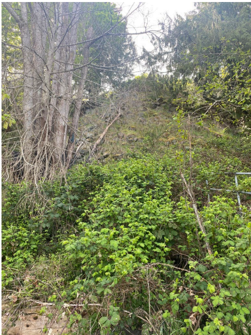
Photo 3.37 Bluff slope with rock armouring that has started to become overgrown with vegetation.
