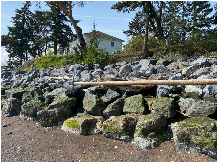
Photo 3.48 Riprap at the southeast end of Protection Island with visible erosion at top of bank. Erosion is suspected to have occurred prior to riprap placement.
