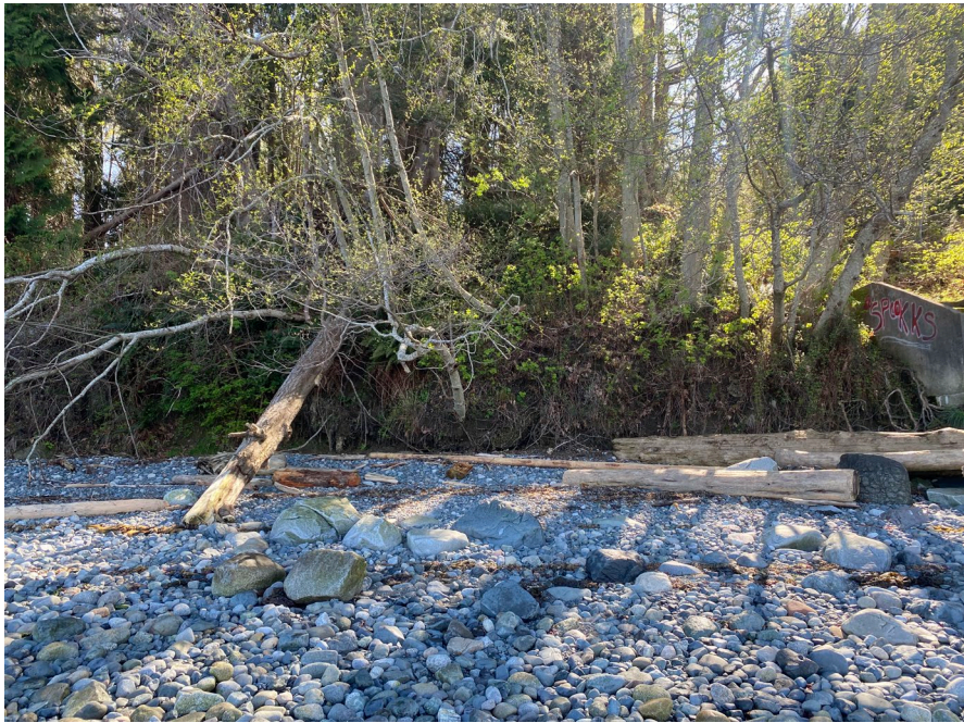
Photo 3.1 Erosion scarp along shoreline
