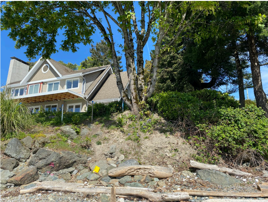
Photo 3.25 Localized area of erosion near Departure Creek
