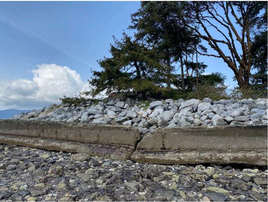
Photo 3.46 Riprap behind failed seawall at southeast end of Protection Island.
