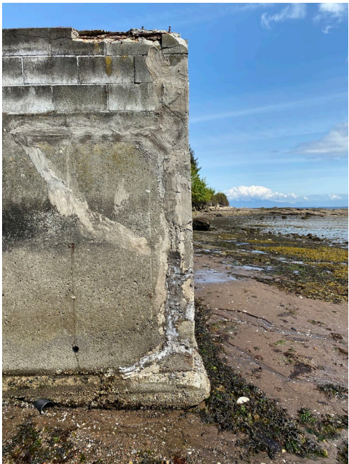
Photo 3.45 Seawall with exposed foundation (~11 inches).
