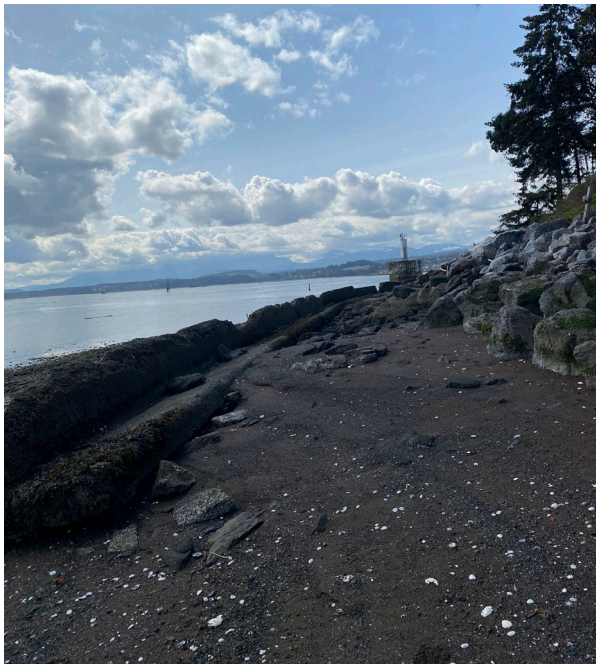
Photo 3.47 Failed seawall and riprap at southeast end of Protection Island with accretion of sand and organics in between
