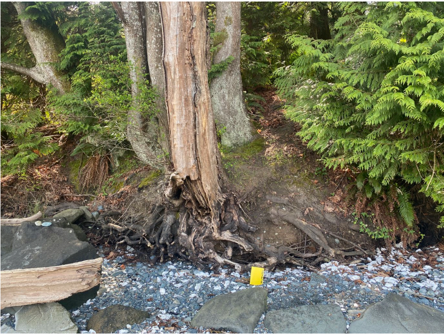
Photo 3.27 Undercutting and exposed tree roots along shoreline.
