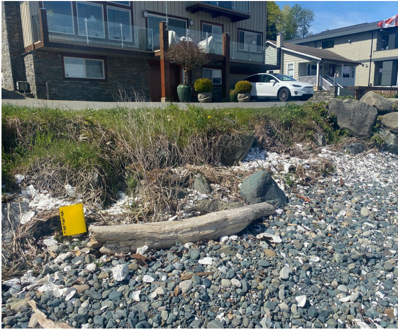
Photo 3.43 Section of Battersea Road where riprap is missing.
