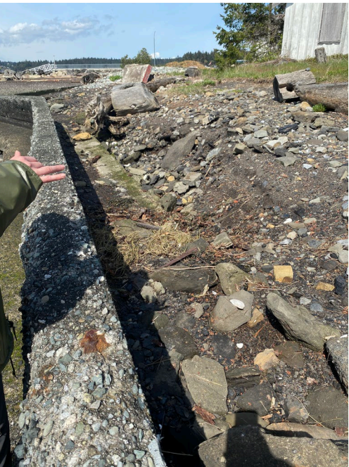
Photo 3.49 Scour behind seawall slabs at south end of Protection Island.
