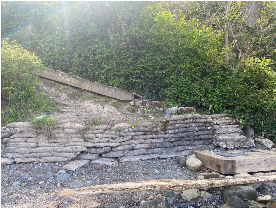
Photo 3.38 Beach access point with sandbags as shoreline protection.
