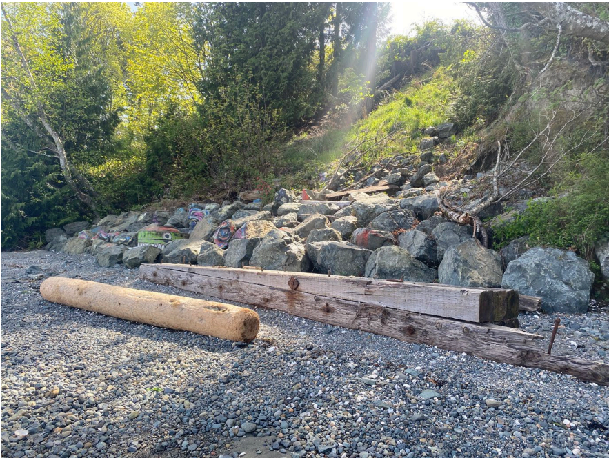
Photo 3.36 Riprap protection along part of the bluff where there appears to have been a slope failure.
