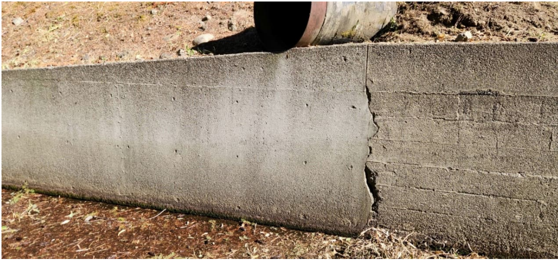
UCR 8: Right Spillway Chute Wall with Crack at Drainage Pipe
