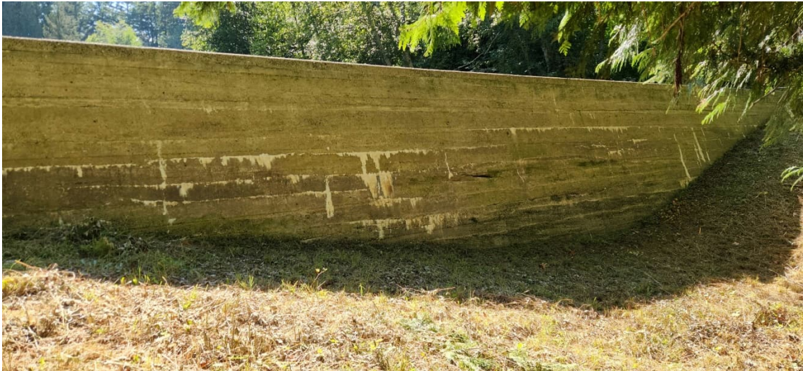
HAW 8: Concrete Deterioration at Downstream Face of the Dam
