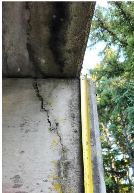
MCR 18: Concrete Crack at Top Corner of Centre Spillway Pier
