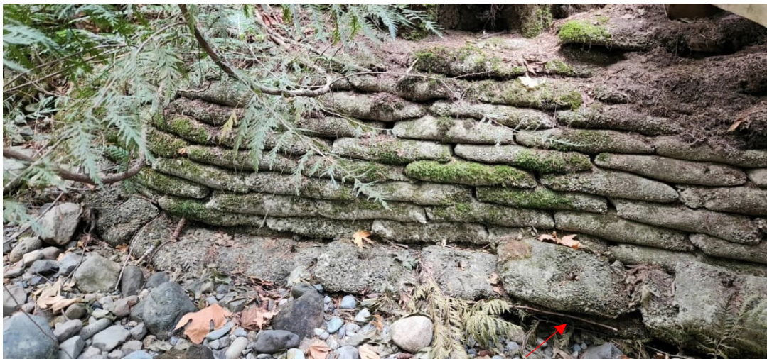
WWL 16: Erosion Damage on Downstream Right Abutment of Bridge (Inlet Channel)
