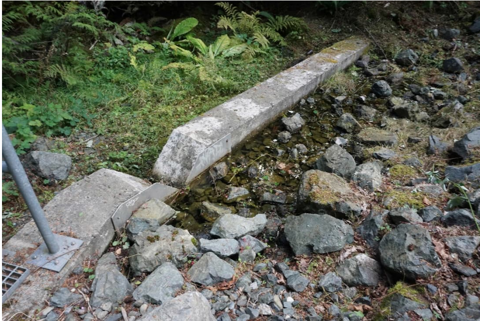
WWL 9: Downstream Seepage Monitoring Weir
