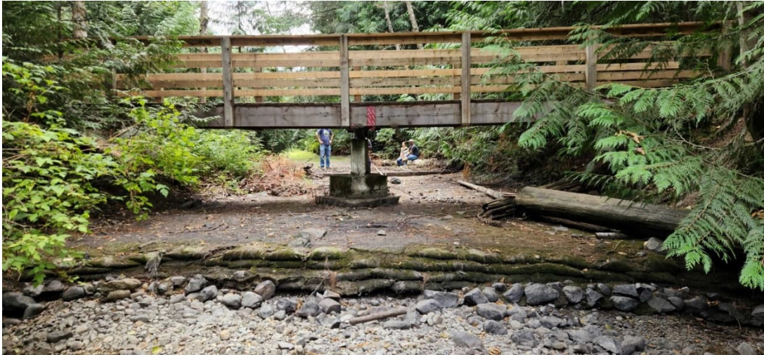
WWL 17: Undermining of the Dam Sacks and Dispersed Riprap at the Downstream Step in the Inlet Channel
