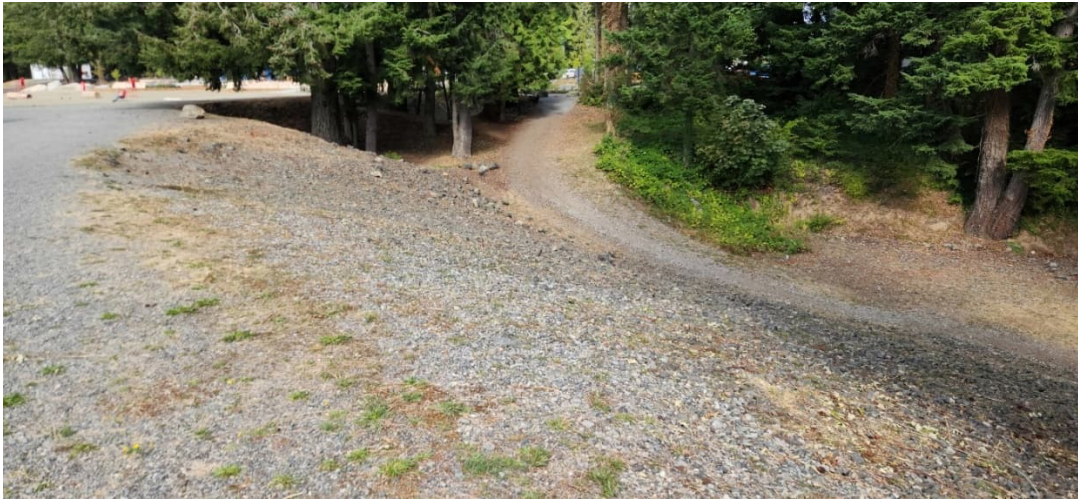
WWL 2: Trees at Crest of Main Dam and Downstream Slope
