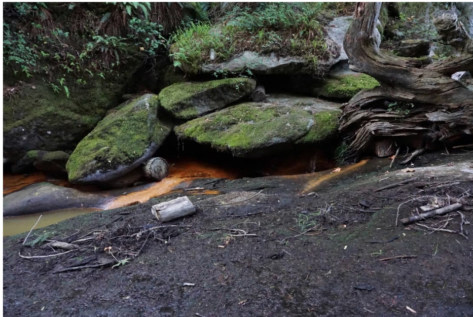
MCR 22: Downstream Seepage
