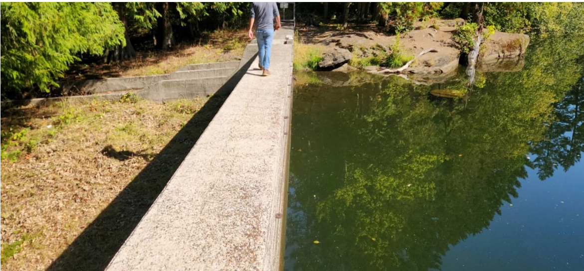
HAW 4: Concrete Deterioration of the Top of the Spillway Bridge
