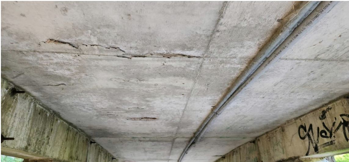
LCR 23: Delamination on Underside of Spillway Bridge
