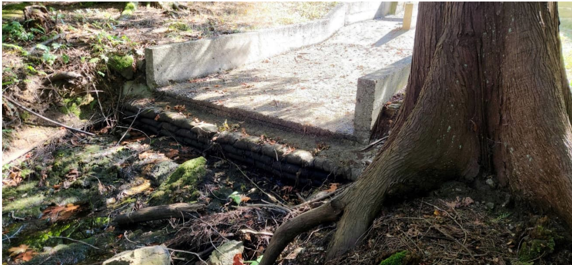
HAW 6: Spillway Slab at Downstream End
