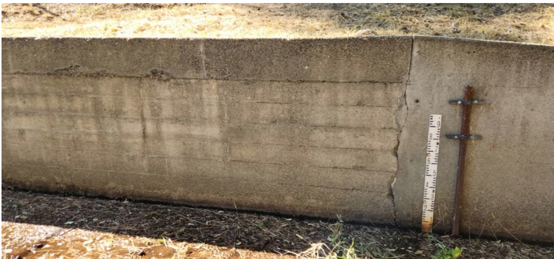
UCR 7: Left Spillway Chute Wall with Crack at Water Gauge
