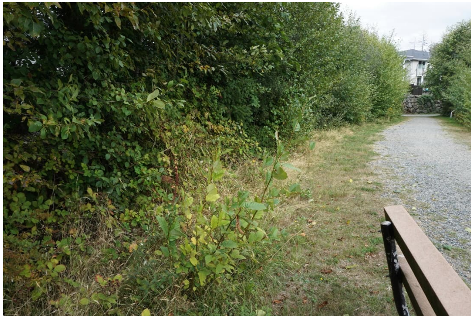
MGC 5: Vegetation on the Downstream Face at Right Abutment
