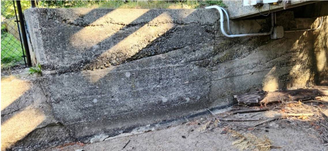
LCR 24: Cold Joints in Left Abutment
