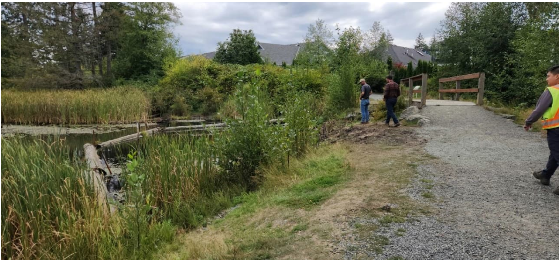
MGC 3: Upstream Slope at Right Side of Spillway
