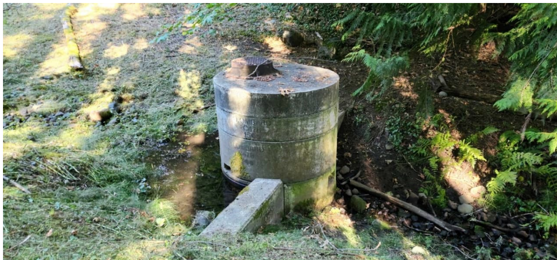
LCR 19: Wet Area at Downstream Toe of Dam and 'V' Notch Weir Housing
