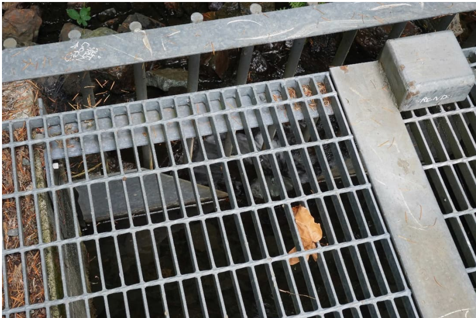
WWL 10: Monitoring weir, looking downstream
