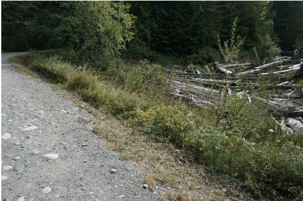
WWL 14: Debris Accumulated at Upstream Toe of Saddle Dam and Light Furrowing on the Upstream Slope
