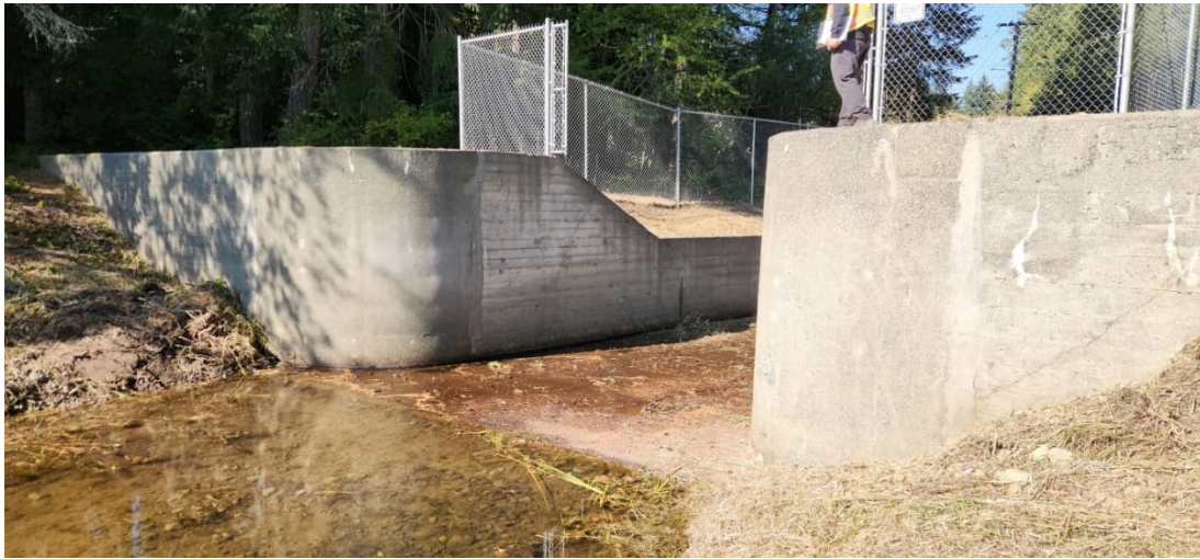
UCR 6: Vegetation Growth Immediately Upstream of the Spillway Channel
