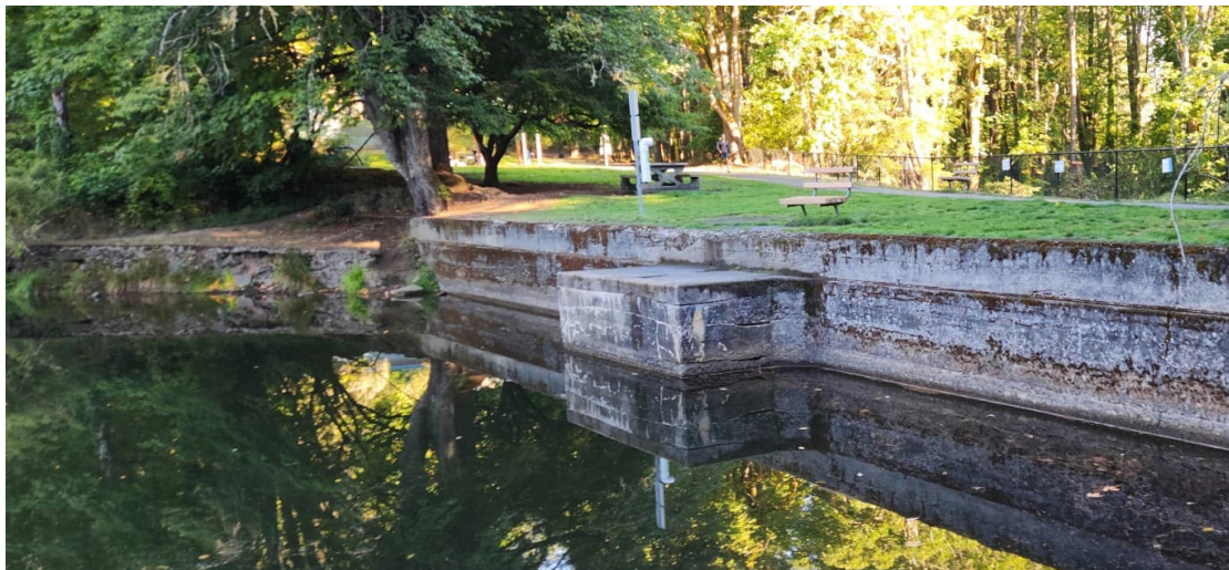
LCR 21: Erosion at Upstream Rock Retaining Rock
