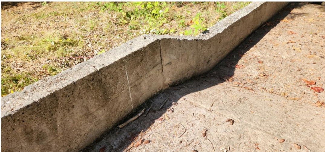
HAW 12: Gap in Joint at Top of Spillway Left Chute Wall
