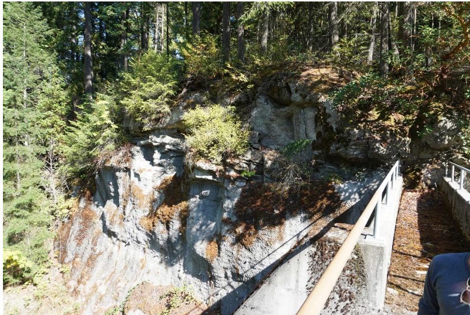
R01 5: Right Abutment Wall Downstream of the Dam (Bedrock, Partially Covered in Shotcrete)
