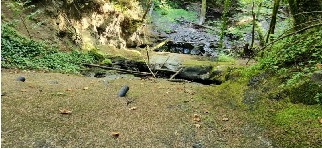
LCR 12: Scoured Rock Channel filled with Debris Downstream of Main Spillway Chute Slab
