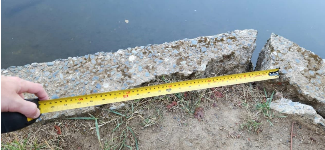
LCR 8: Cracks at Upstream Lower Wall Corner
