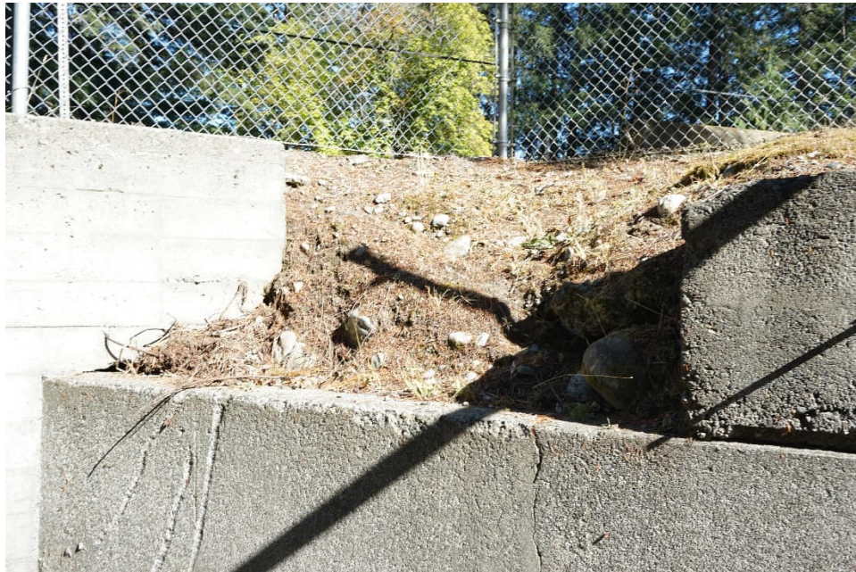
UCR 12: Surface Runoff Erosion Along Wingwall Slopes
