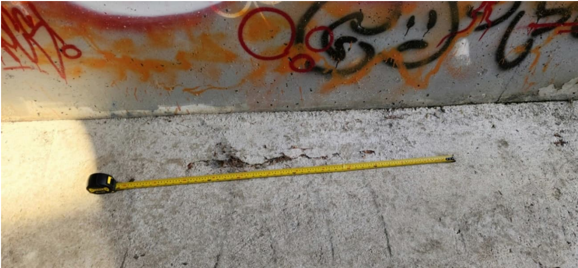
LCR 25: Delamination by Right Wall of Auxiliary Spillway
