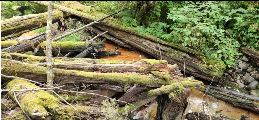
WCL 1: Left Abutment of Dam Showing High Degree of Deterioration
