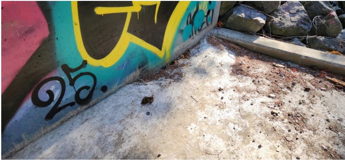
LCR 26: Spall at Left Wall of Auxiliary Spillway
