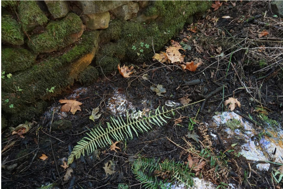
HAW 15: Small Seepage Area Downstream of the Rock Wall
