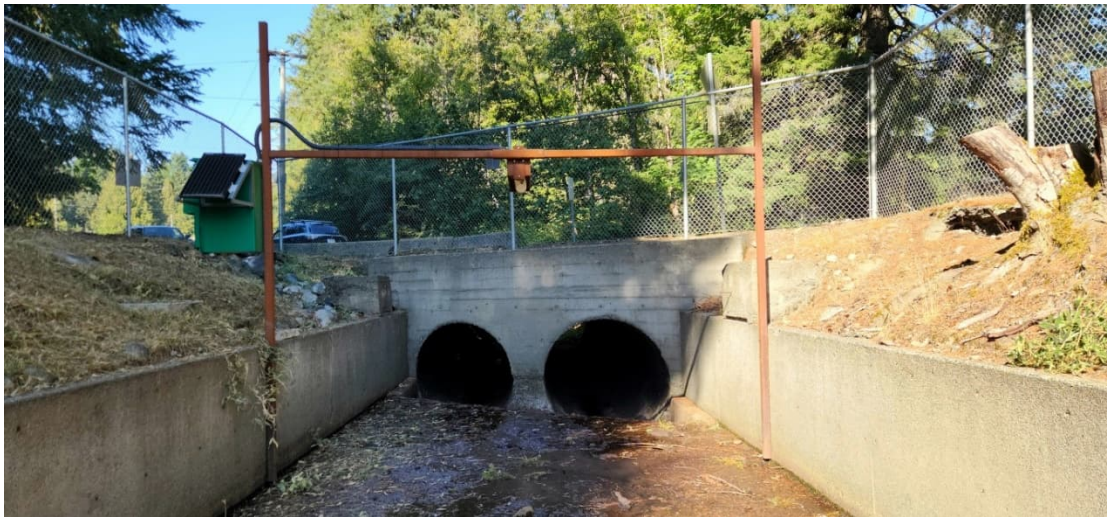
UCR 13: Surface Runoff Erosion Along Wingwall Slopes
