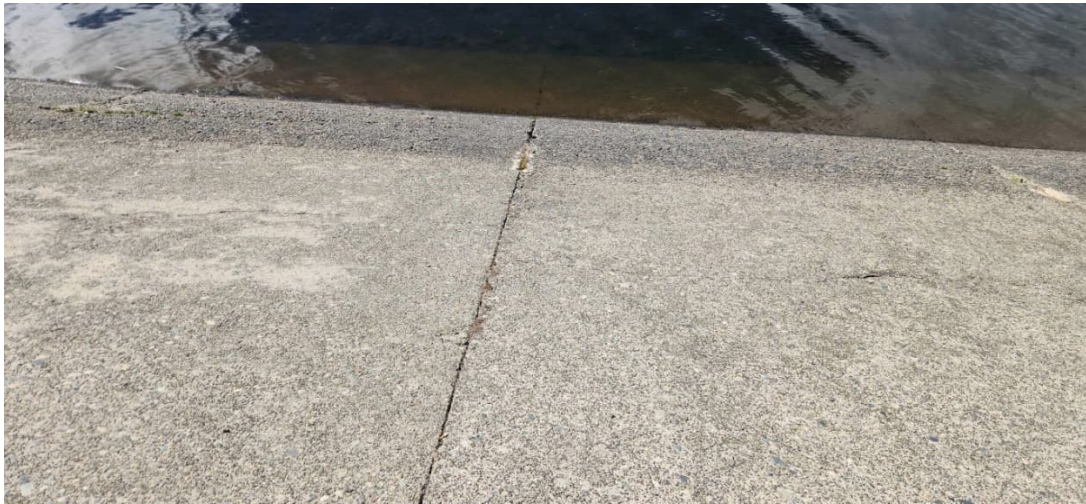
WWL 3: Upstream Concrete Face of Main Dam with Horizontal Cracking
