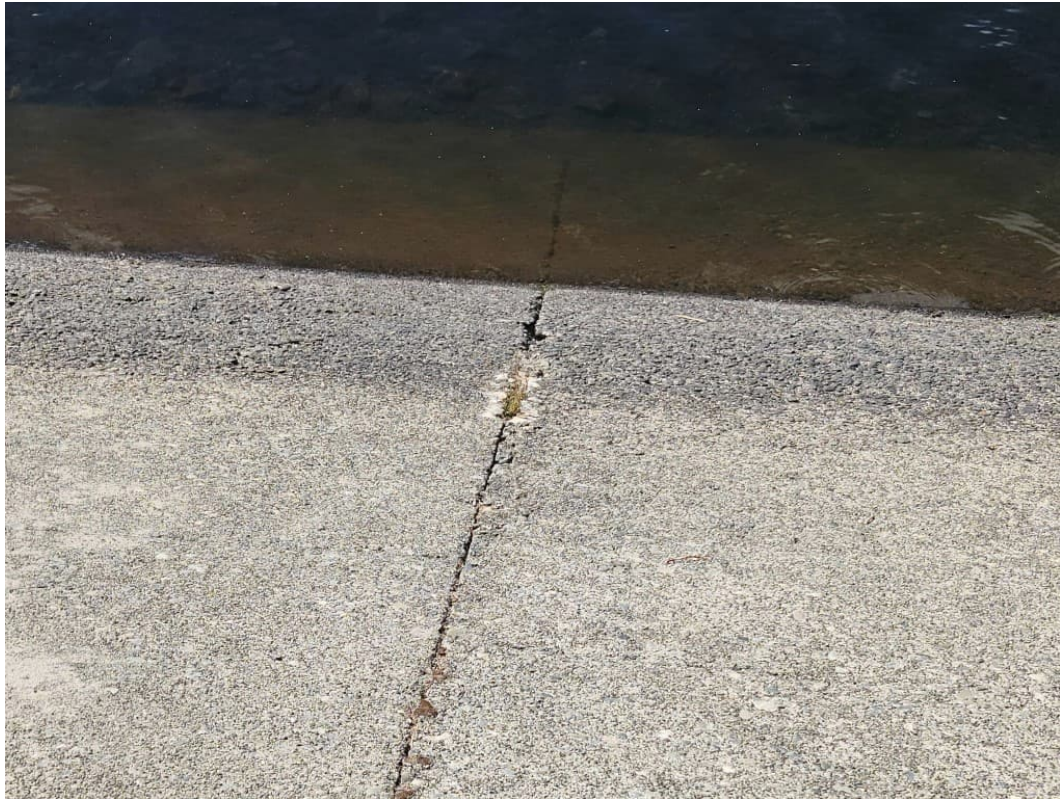
WWL 4: Upstream Concrete Face of Main Dam with Joint Deterioration and Cracking
