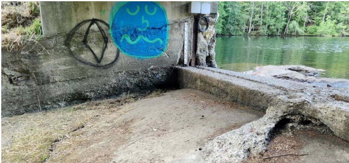
MCR 20: Undermining of Right Abutment Wall
