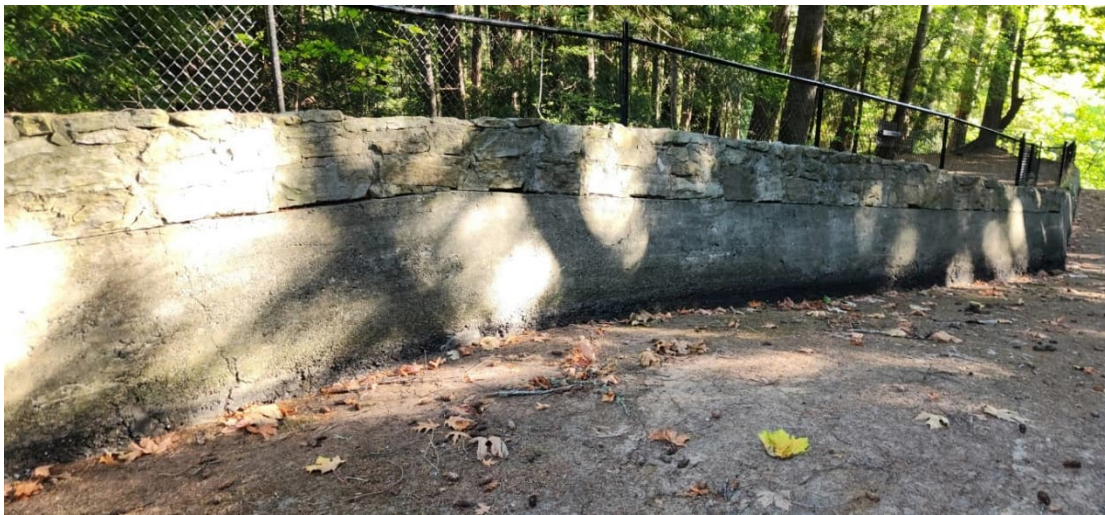
LCR 9: Erosion at the Base of the Spillway Chute Left Concrete Wall
