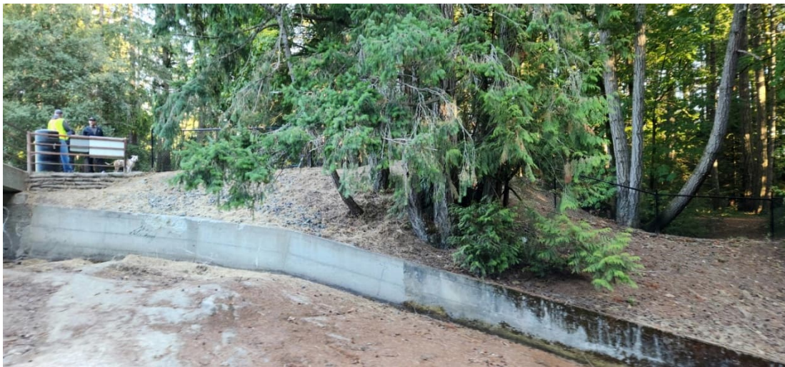
MCR 16: New Fence/Handrail and Presence of Cobble Cover at Left Side of Spillway
