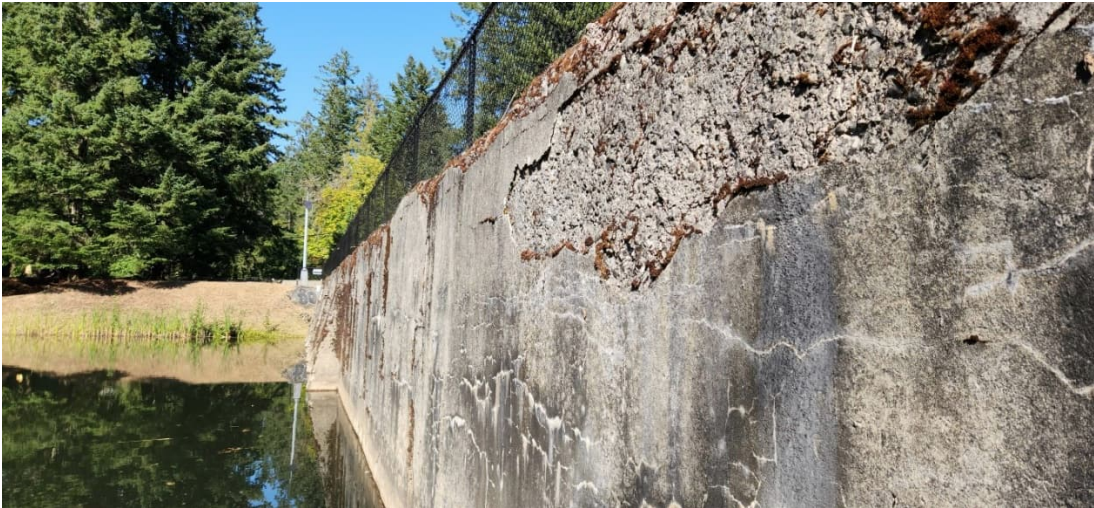
UCR 3: Concrete Deterioration at Right Side of Buttress Wall of the Dam
