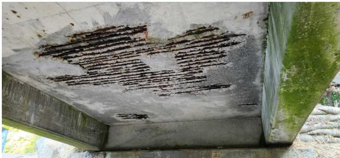
MCR 4: Concrete Deterioration with Exposed Reinforcing Bars Underside of the Spillway Bridge Deck (Left Bay)
