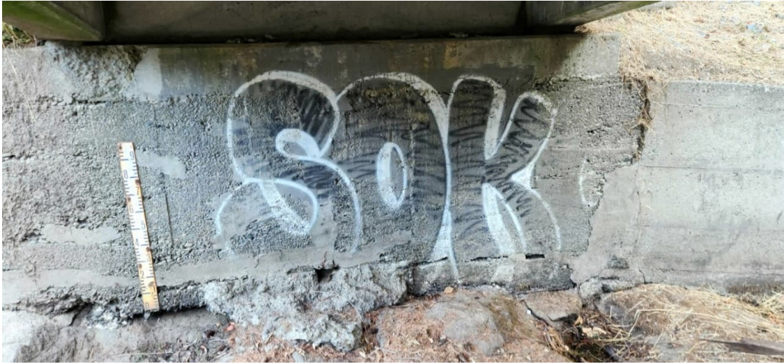
MCR 21: Undermining of Left Abutment Wall
