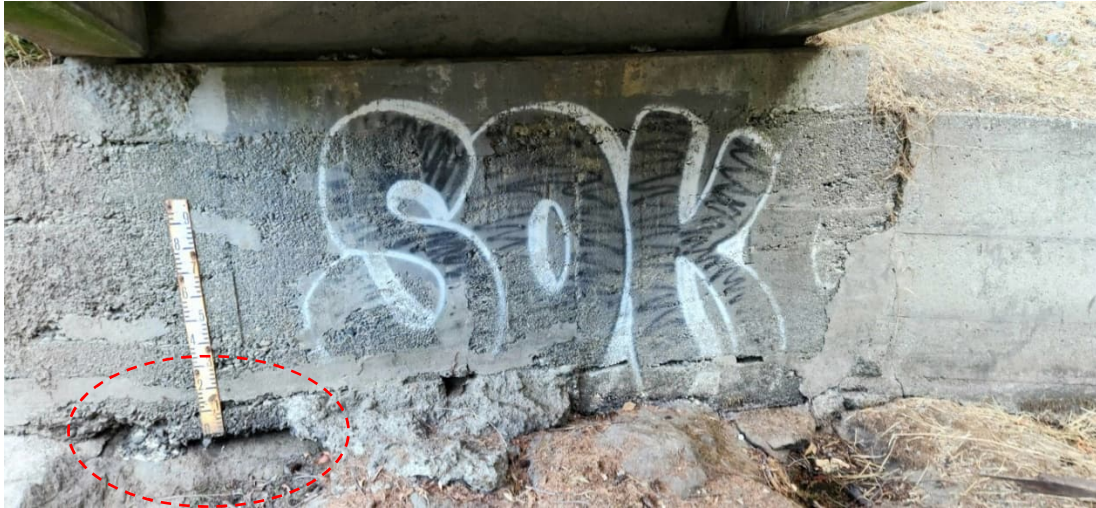
MCR 5: Concrete Erosion at Contact with Rock at Left Abutment of the Spillway Bridge Deck (Left Bay)
