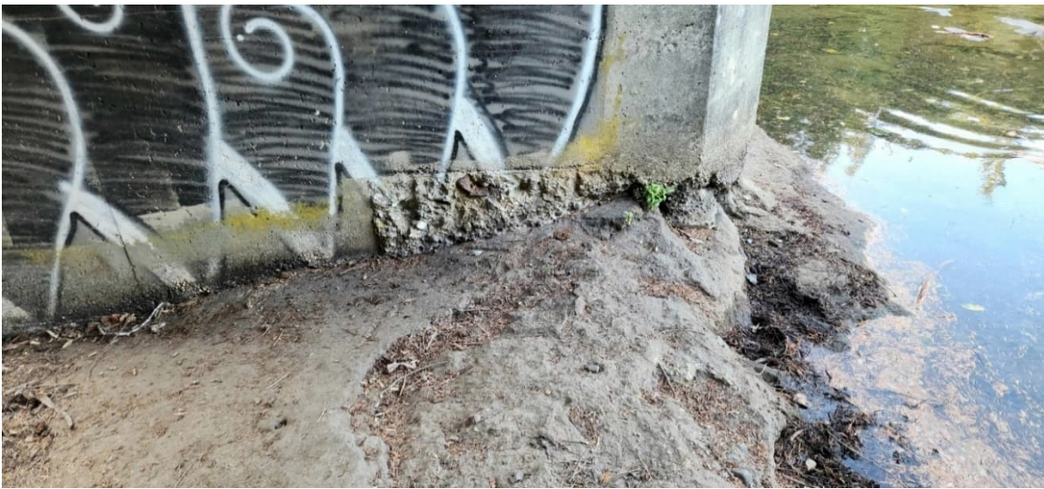
MCR 19: Undermining of Central Spillway Pier
