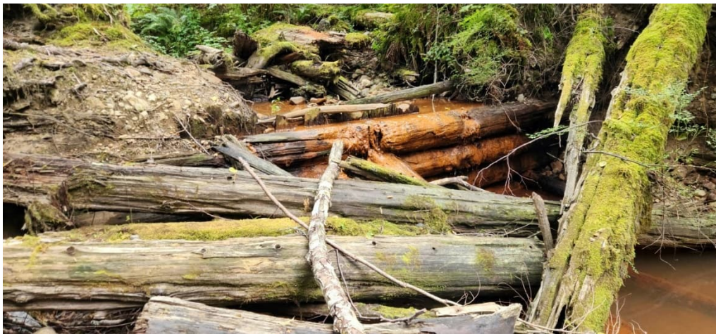
WCL 3: Dam Showing High Degree of Deterioration
