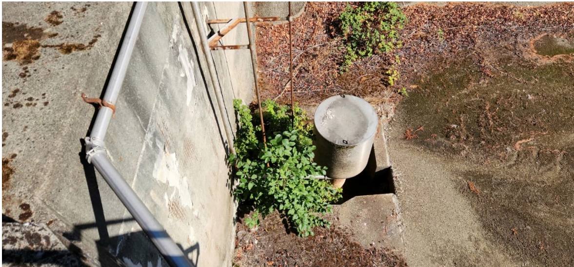
R01 4: Mechanical Equipment at Upstream Side of the Dam
