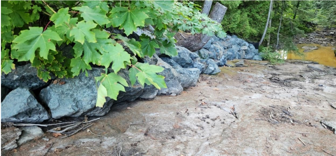
MCR 15: Newly Placed Riprap at the Left Embankment Beyond the Wing Wall
