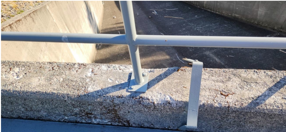
JCR 43: Spalling on Bridge Curbs
