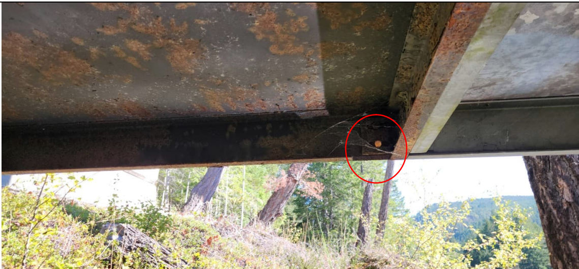
SFK 18: Missing Fasteners on Inlet Operating Platform
