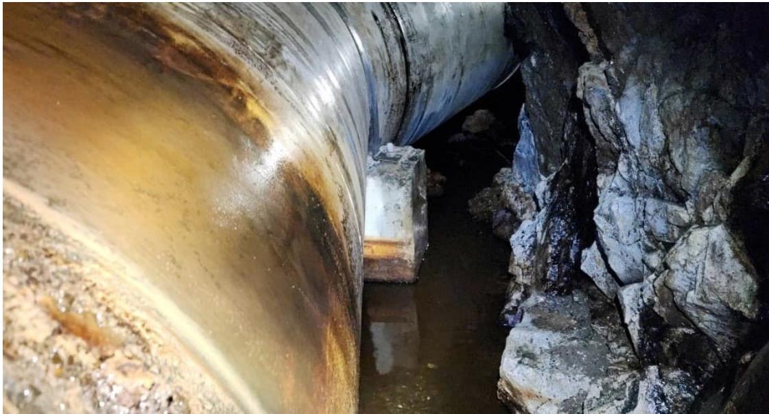
SFK 9: Water Supply Pipe Anchor and Foundation Block
