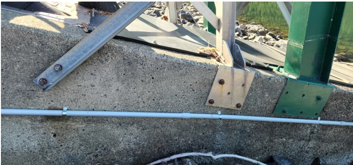
JCR 46: Corroded Fasteners on LLO Operating Platform
