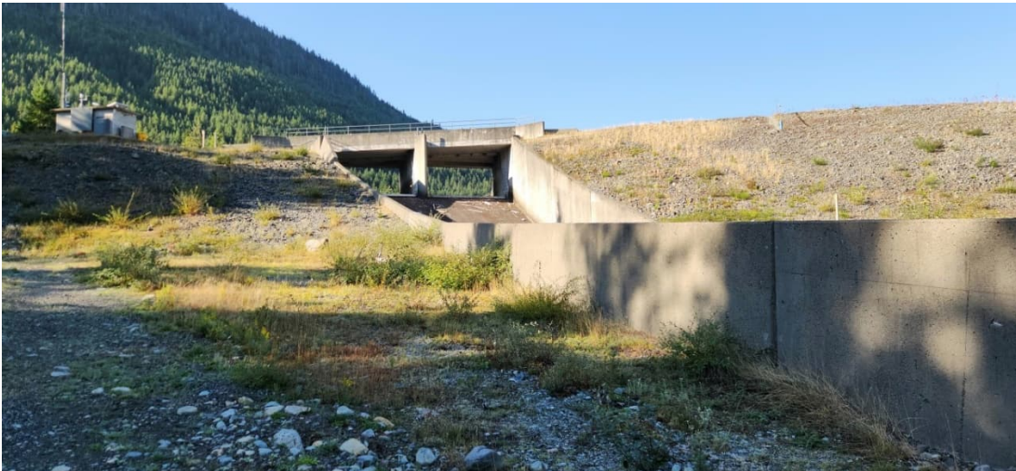
JCR 10: Vegetation near to Right Wall of Spillway Chute
