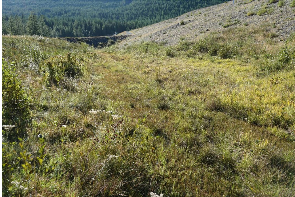
JCR 33: Downstream Toe with Ruts and Seepage
