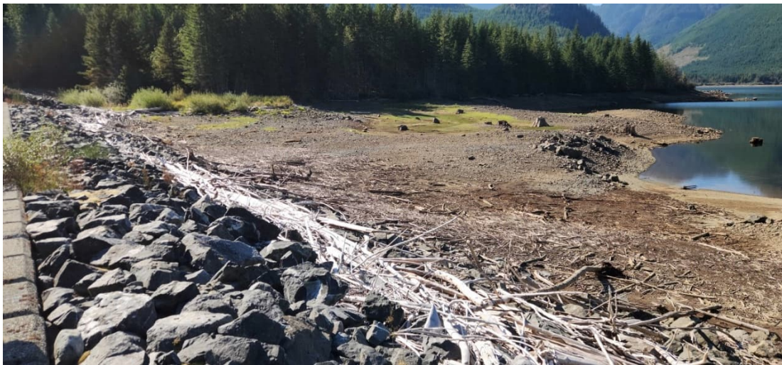
JCR 34: Auxiliary Spillway with Concrete Block Crest and Upstream Face of Dam (Looking towards the Right Abutment)
