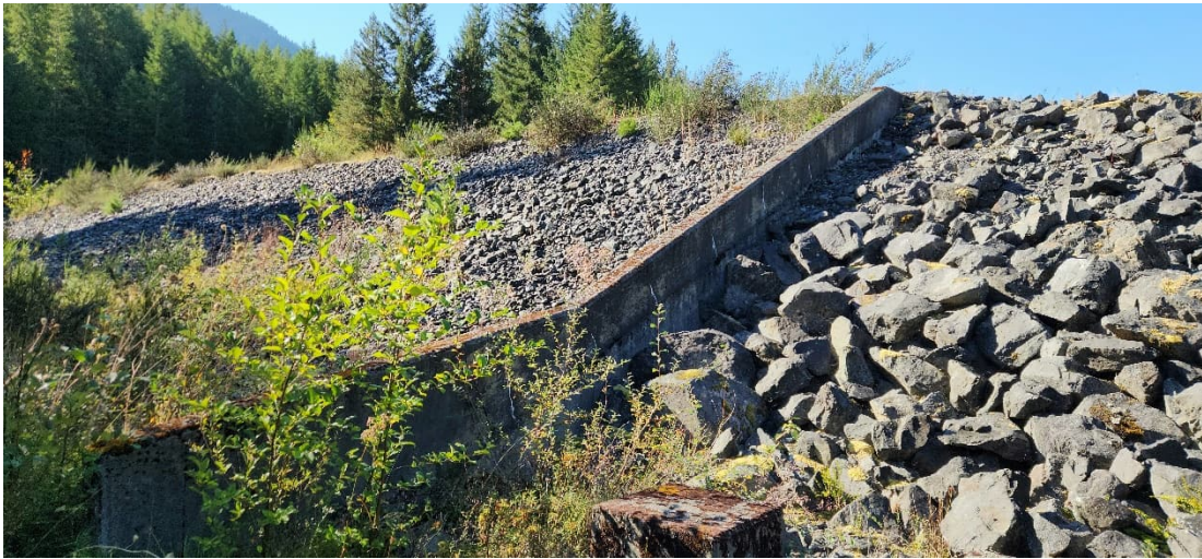
JCR 36: Auxiliary Spillway and Downstream Face of Dam, zone with sparse riprap
