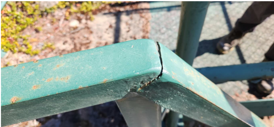
SFK 16: Broken Weld on Handrail at Inlet Operating Platform
