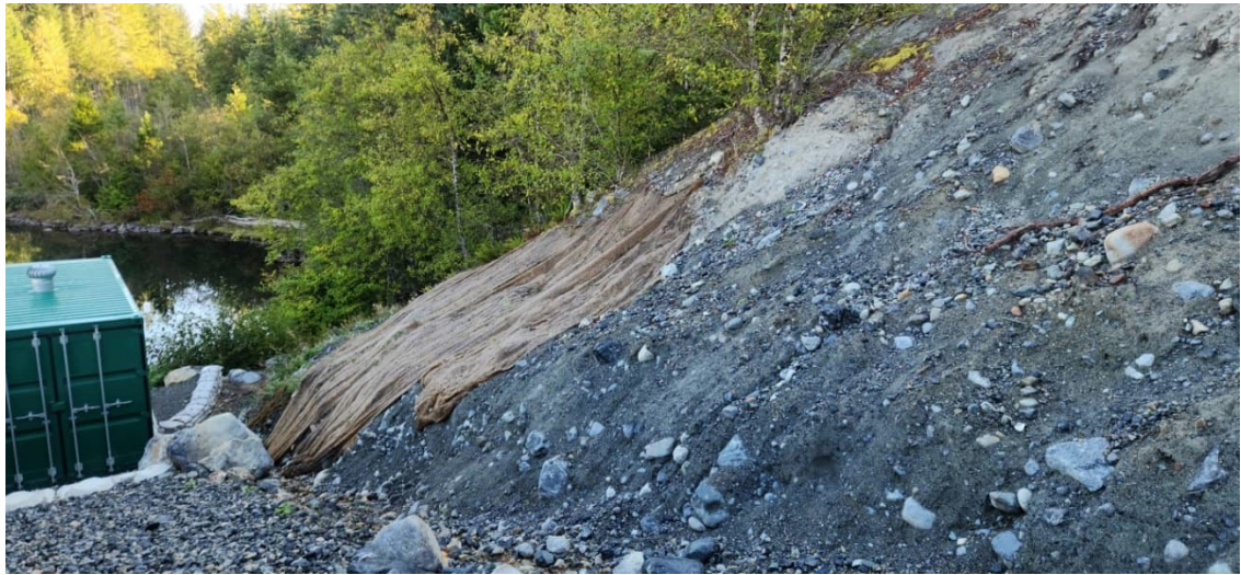
JCR 42: Erosion by Turbines
