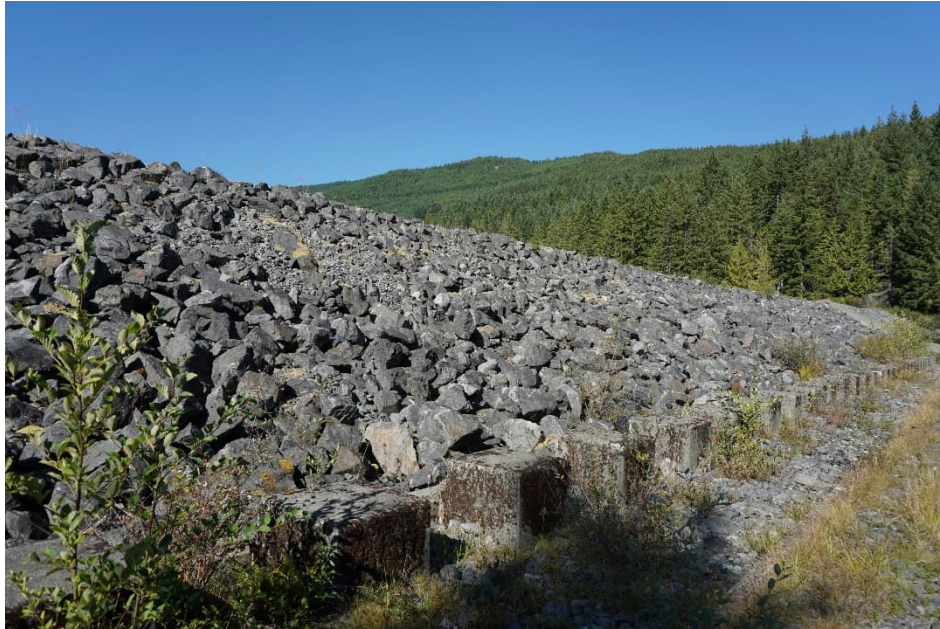
JCR 37: Auxiliary Spillway and Downstream Face of Dam, zone with sparse riprap
