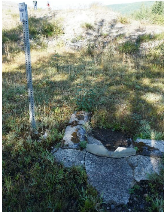
JCR 29: Flowing Water at Weir E
