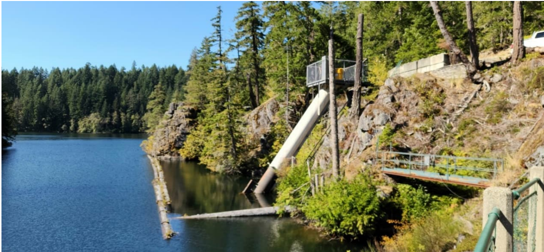
SFK 4: Water Supply Intake Debris Boom
