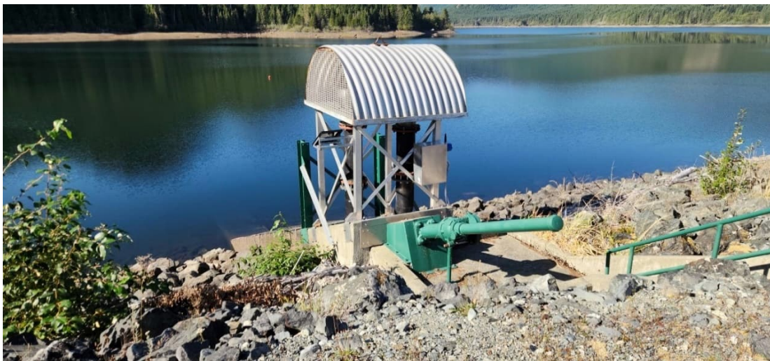
JCR 6: LLO Intake Gate at Upstream Face
