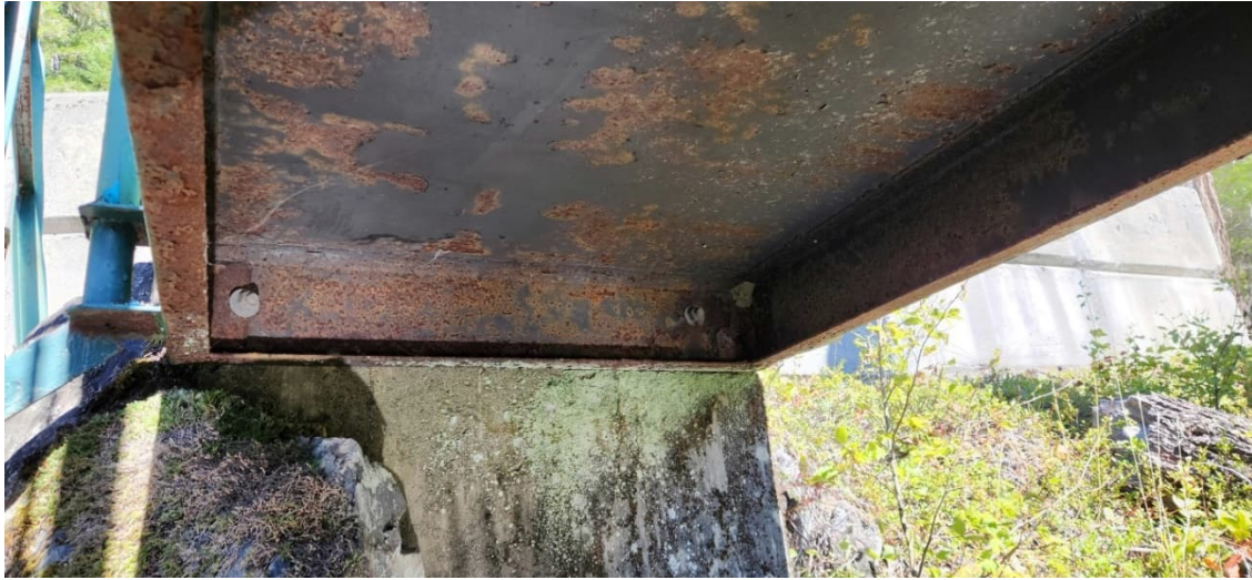
SFK 17: Corrosion on Underside of Inlet Operating Platform Ramp
