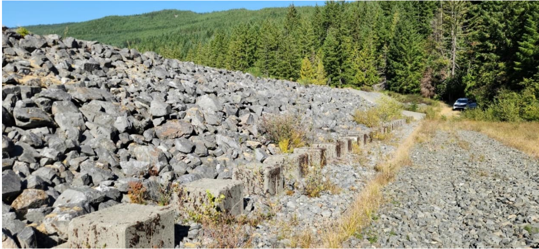
JCR 35: Auxiliary Spillway and Downstream Face of Dam (Looking towards the Left Abutment)
