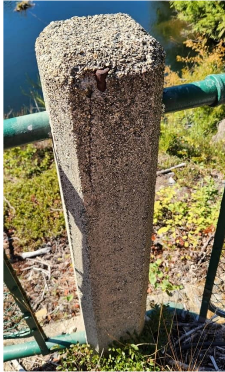
SFK 15: Handrail Post with Exposed Reinforcement
