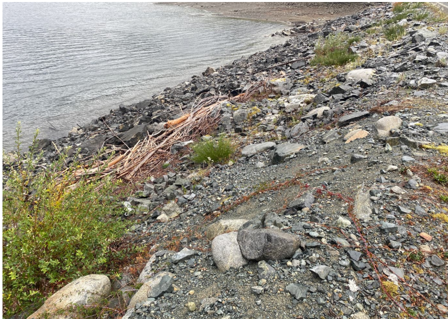
JCR 30: Poor Quality Riprap Left of Piezometer SP12
