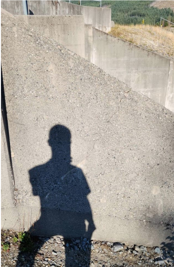
JCR 44: Cracking on Right Abutment Wall
