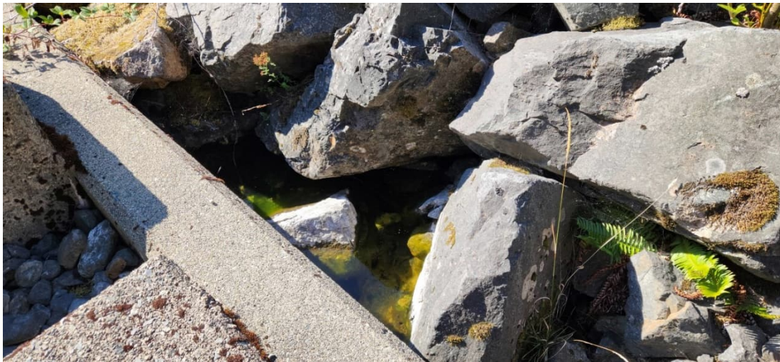
JCR 38: Seepage at Downstream Toe of Auxiliary Spillway
