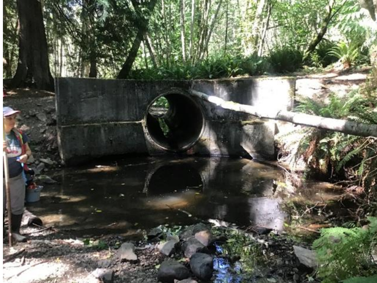
Figure 8. The 200 Linley Road culvert is impassable to fish and large organic material (barrier between Reaches 3 and 4).
