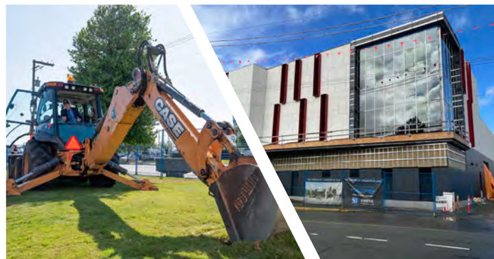
Construction of the new Fire Station #1 has come a long way! It is nearing completion with an official opening expected to take place later this fall.
