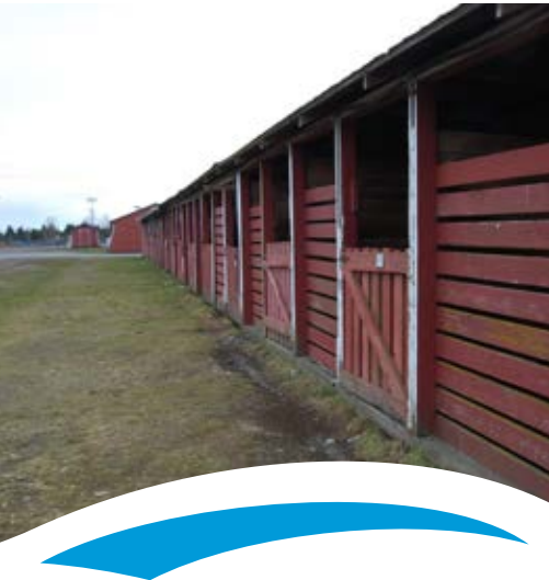
Stalls and barns in the centre of Beban Park are in poor condition.
