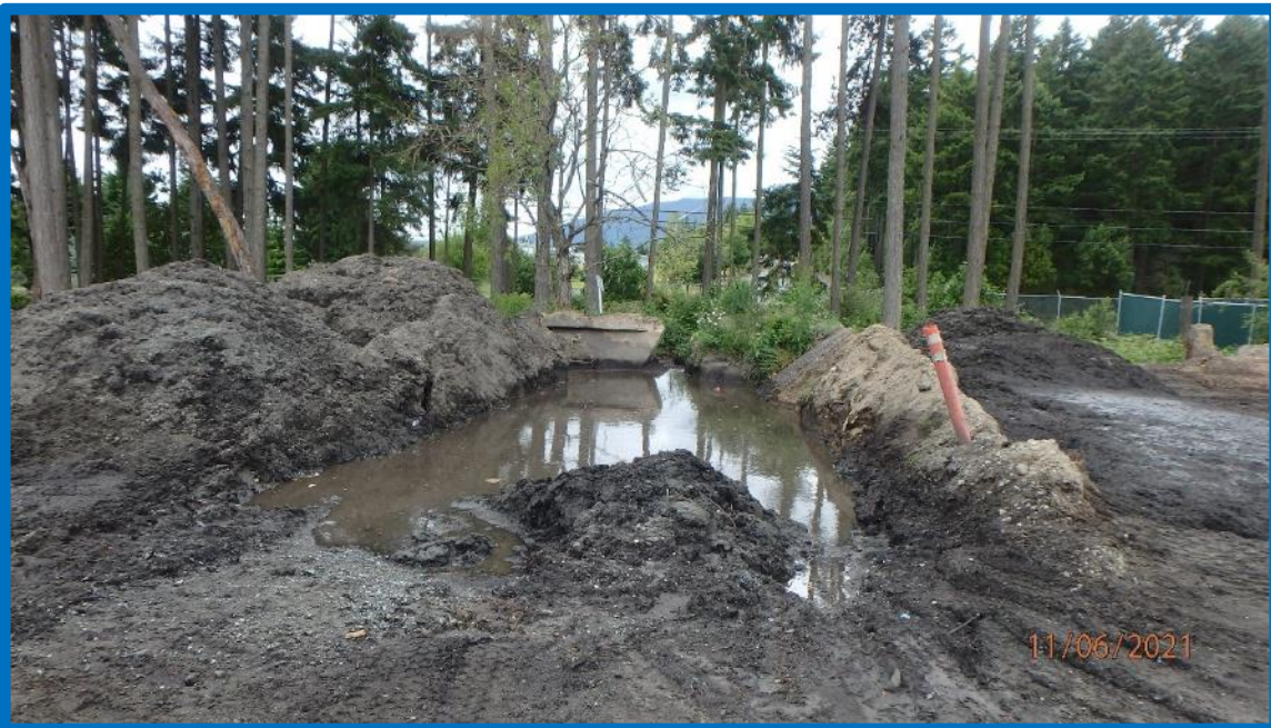
Image 18 Vacuum Truck Dewatering Area
