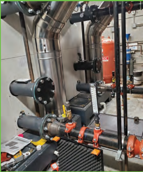
New, more efficient boilers installed in NAC
